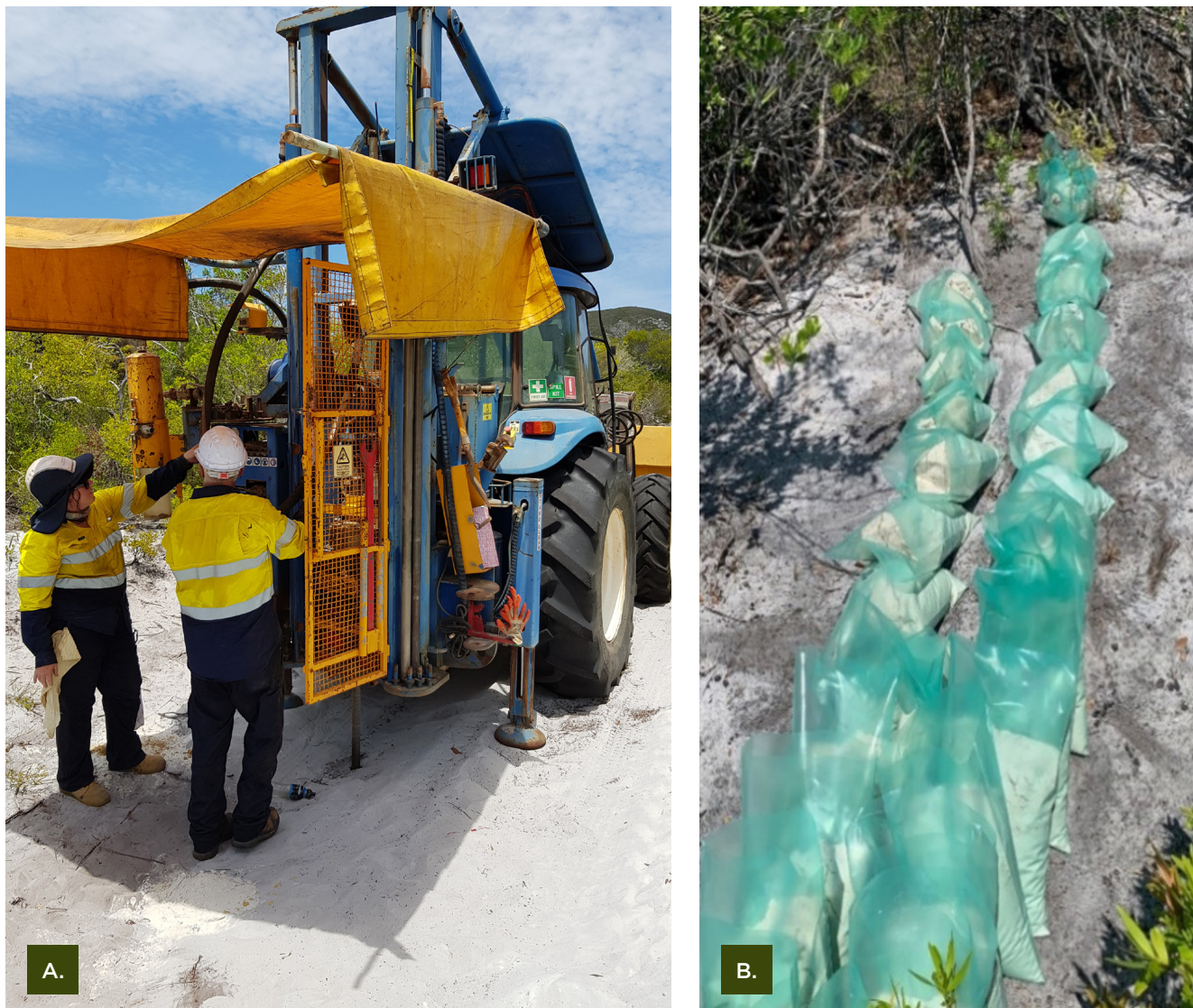
Figure 9: A. A vacuum drill rig in operation at site, and B. Collected and bagged sand samples
